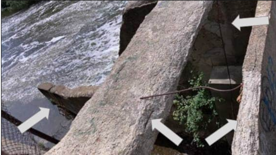
Figure 9. Exposed reinforcing steel in auxiliary spillway.
