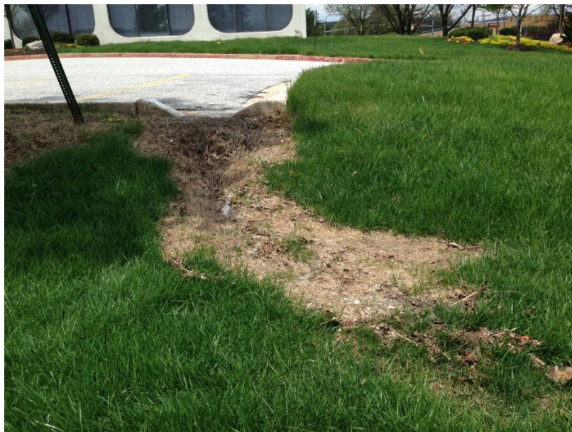
Figure 1 - Roadside grasses and other vegetation can be killed off by road salt. These plants are important for preventing soil erosion. All types of vegetation, even trees, can be killed off, or at least weakened, by road salt when they are coated in it due to spray from traffic, or by taking up salty snowmelt through their roots. Source: Sustainable Stormwater Management.
