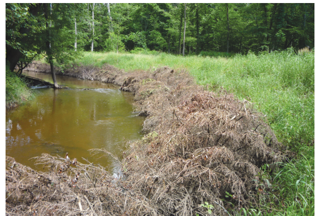
After streambank restoration. Nearly one year after construction and high flows, the banks are vegetated with native trees, shrubs and grasses.
