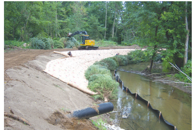
During. Crews pull back the slope and install soft engineering techniques such as erosion control blankets and trees sourced from a local tree farm. Photo: ECT
