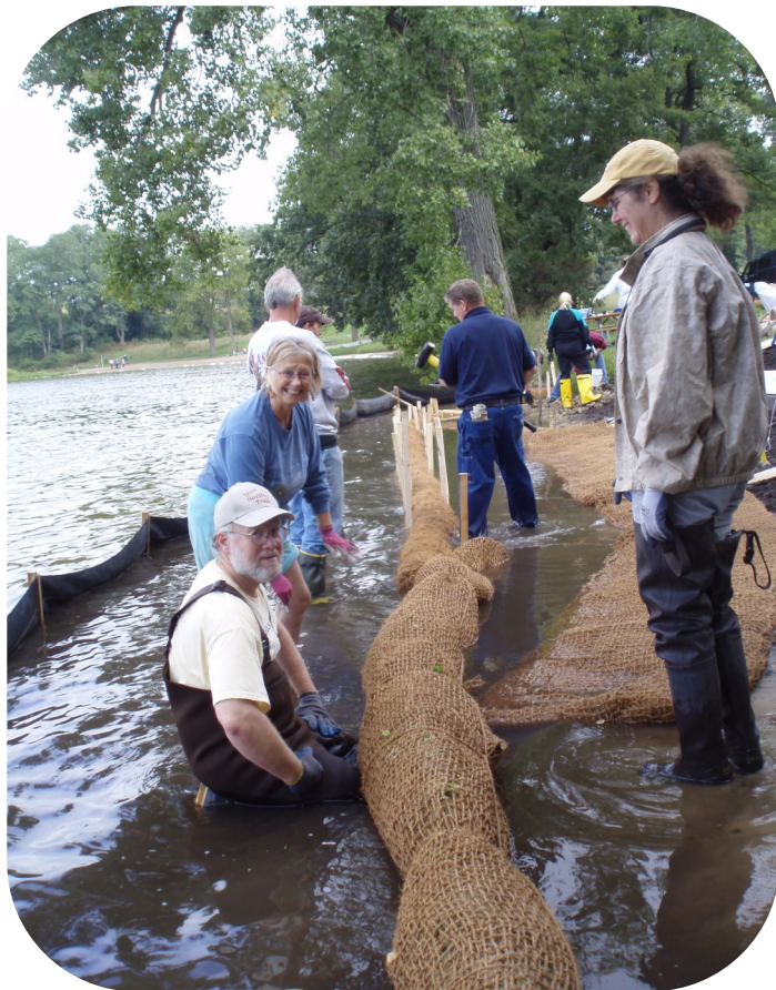
Volunteers installed natural shoreline protection at two sites along Bishop Lake in the Chilson creekshed. Credit: Michigan DEQ.
