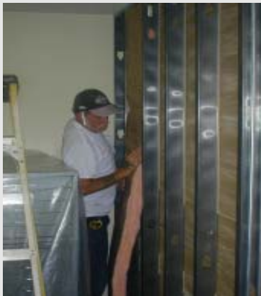
Modification of the new office space, labor and materials donated by McKinley Associates. — photo: HRWC
